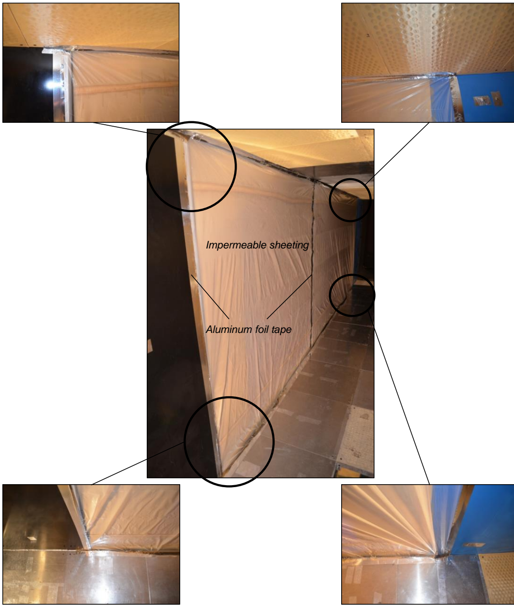
FIGURE 5.19. Sealing of the port chamber with plastic sheeting. Foil tape was used to seal the edges all the way around the Kevlar including the four corners as detailed above. Two sheets have been joined with foil tape towards the center of the Kevlar wall.
