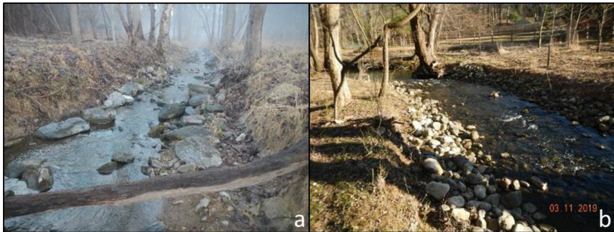
Figure 3.21 Two examples of constructed riffles that included armor on the adjacent banks. Constructed riffle from restoration project 10 that is experiencing bank erosion on the adjacent banks, despite large rocks that were placed to provide armoring (a). Constructed riffle from restoration project 18 that utilized the same substrate to construct the riffle and the bank armor (b).
