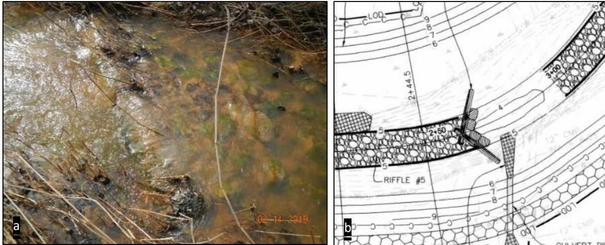
Figure 3.49 Log full span vane at restoration project 9, where the left arm is completely buried (a). The design drawing for the structure is provided in (b).
