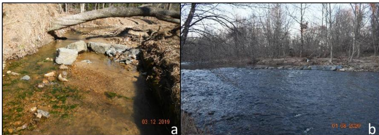
Figure 3.17 Two examples of rock j-hooks, including the sill portion of a j-hook from restoration project 28 (a) and a large j-hook from restoration project 35 where the sill is submerged (b).
