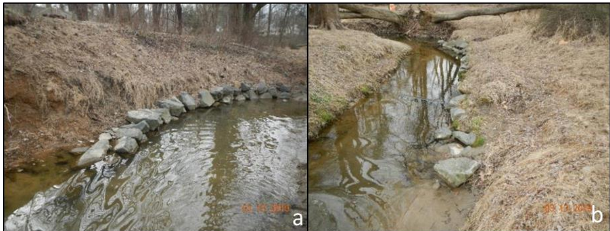
Figure 3.57 Two stone toe structures from restoration project 33. Both structures illustrate that the ends of these bank protection structures are compromising structure function. The structure in picture (b) is experiencing bank erosion on both ends.
