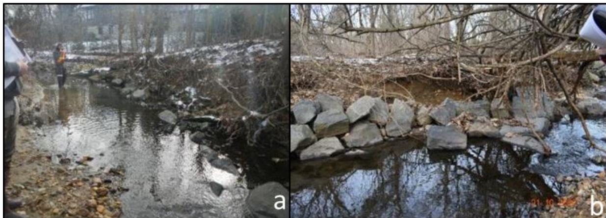
Figure 3.55 Two bank protection structures from restoration project 7 that illustrate how overtopping contributed to structure degradation. In both cases, the bank above the structure is eroded and the structure is destabilized.
