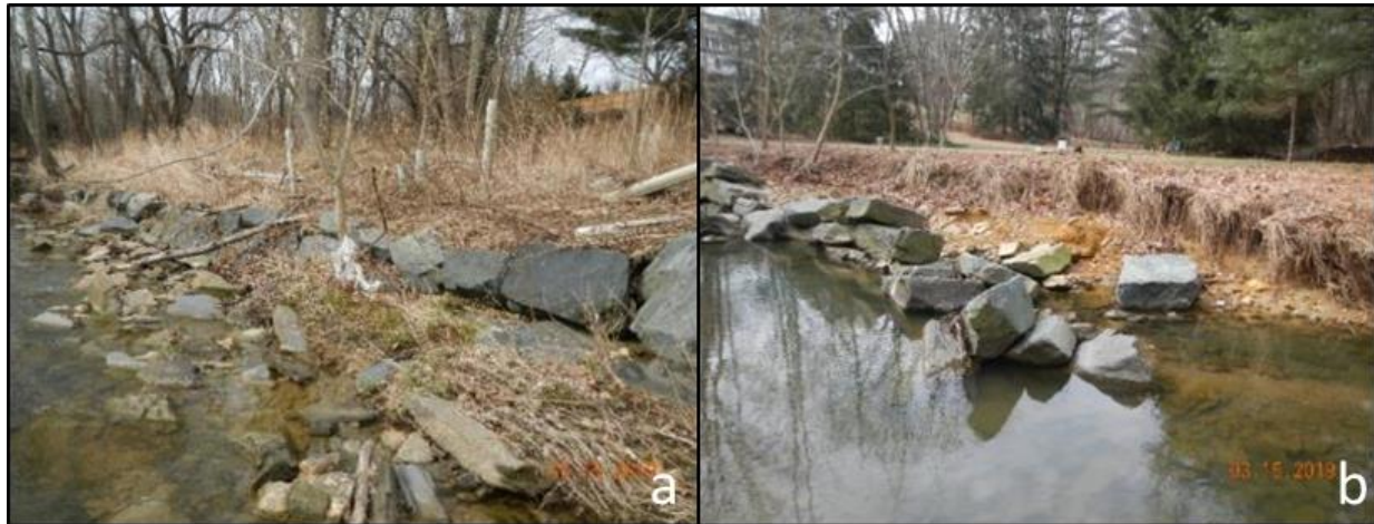
Figure 3.56 Two examples of BP structures from restoration project 24, one that is functioning (a) and one that is failing (b). The failing rock wall is the downstream end of a longer structure, and failure seems to have stemmed from overtopping leading to structure destabilization.
