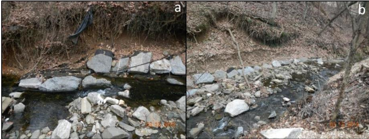
Figure 3.58 Two bank protection structures from restoration project 12 with erosion above the structures.
