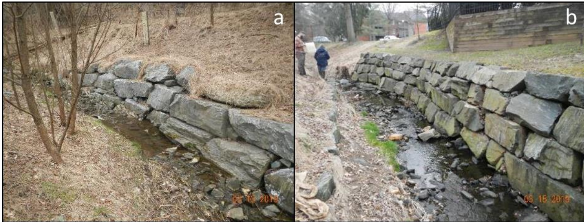
Figure 3.1 Two examples of imbricated rock walls from restoration project 1 (a) and 4 (b), respectively.
