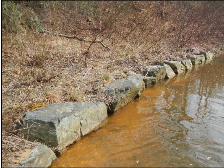
Figure 3.60 Example of stacked rock toe from restoration project 9. Although not visible in this photograph, there is a layer of footers below the stones.
