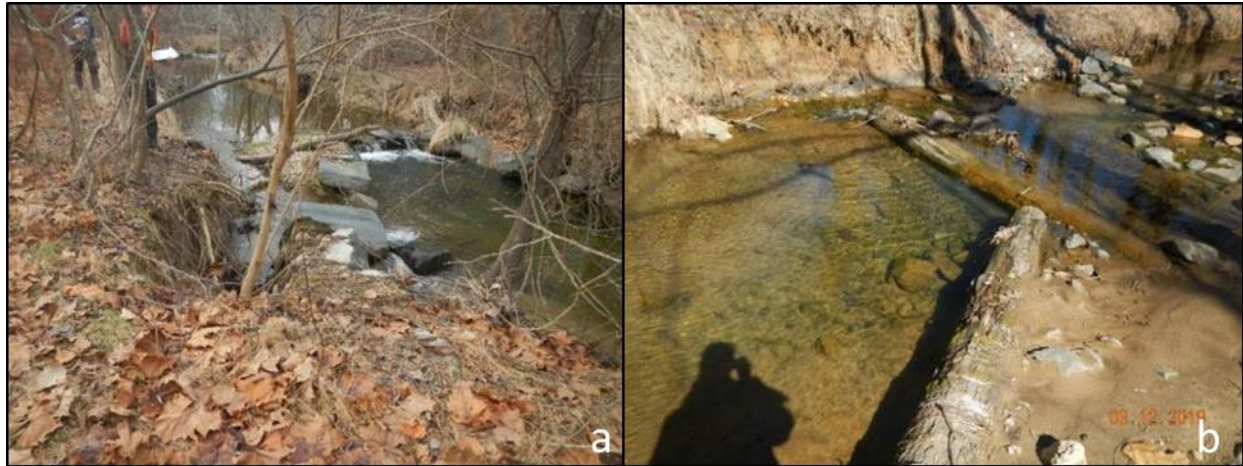
Figure 3.11 Two full span vanes that failed due to flanking. a) shows a rock cross vane from restoration project 31; b) shows a log cross vane from restoration project 28, which is missing the entire right arm.
