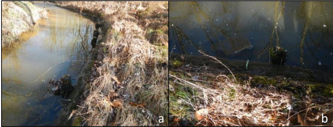
Figures 3.33 Log toe structure on the right streambank (a) and log toe with exposed rebar and visible wood piles (b). Both images are from restoration project 36.
