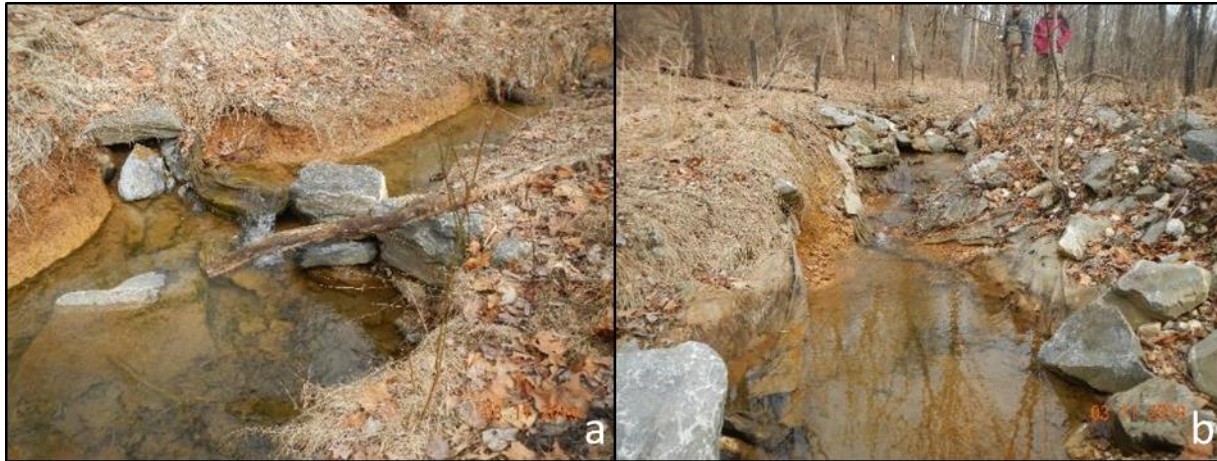
Figure 3.10 Examples of a knick-point and resulting structure failure from restoration project 8. A full span vane that failed due to the migration of a knick-point, such that the structure is now above the current baseflow water surface elevation and structure materials were displaced into the downstream pool (a) and the downstream reach that was affected by this knick-point (b).
