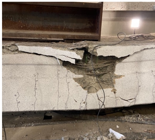
Figure 5.23. Concrete Crushing Failure Mode
