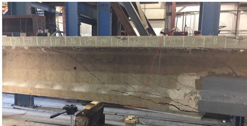
Figure 5.15. Flexural Shear Failure of the HRBT Beam Repaired with CFRP
