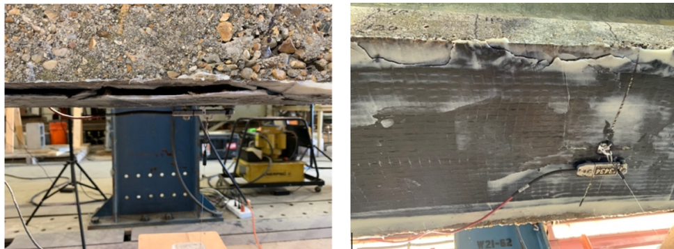
Figure 5.14. CFRP Debonded from the Soffit of the HRBT Beam
