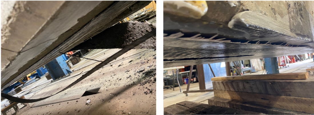
Figure 5.22. CFRP Debonded and Ruptured on Bottom of Box Beam
