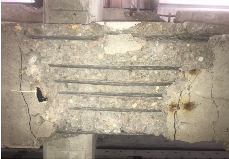
Figure 3.6. Bottom of I-Beam 7 after Testing
