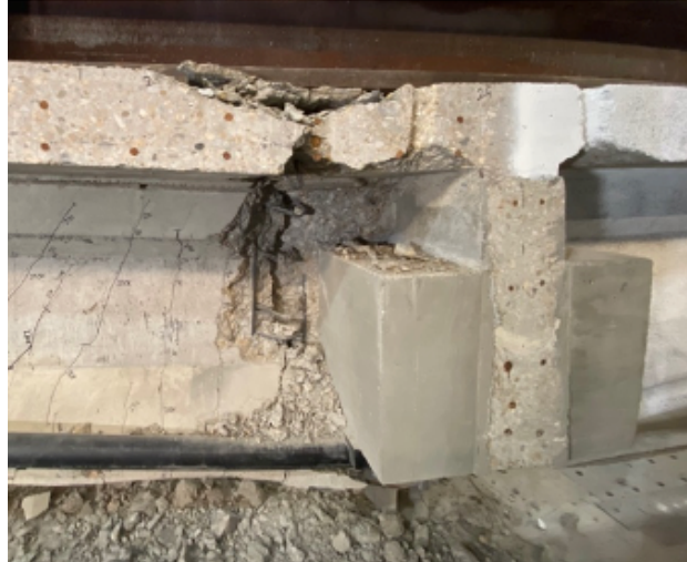
Figure 4.13. Concrete Crushing at the Top of the Beam – I-Beam 1 - Repaired with External PT – Wax
