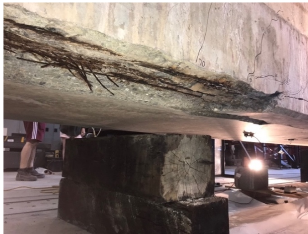
Figure 3.10. Three corroded strands in Box Beam 1
