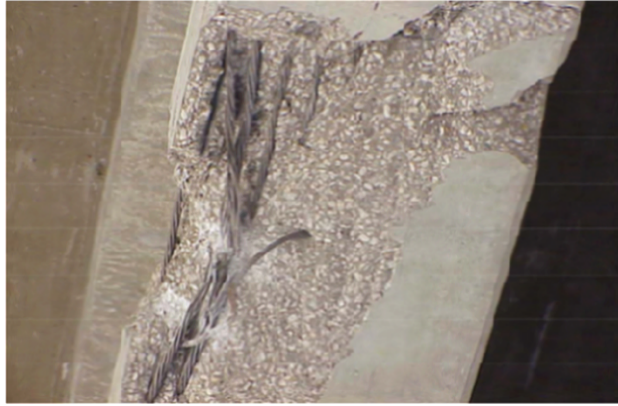
Figure 2.17. Signs of damage in the tested beam (Klaiber et al., 2003)
