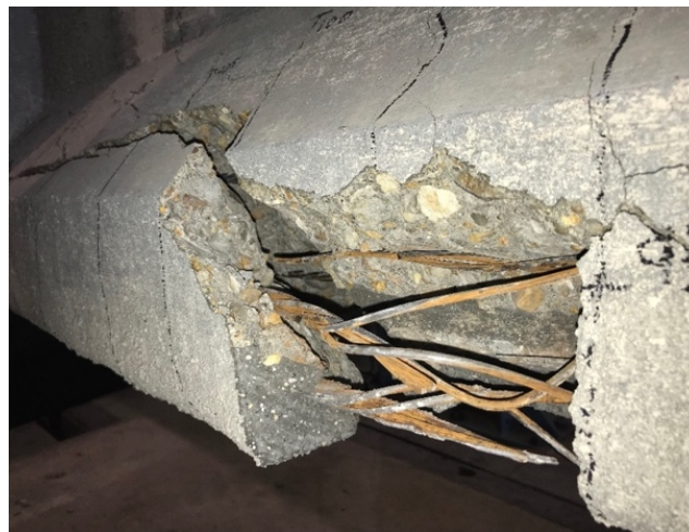
Figure 3.8. Corrosion-Damaged Strands in and above Patch in I-Beam
