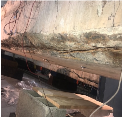
Figure 3.13. Corroded Strand on Bottom of Box Beam 2
