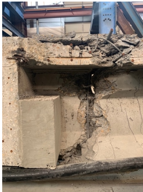
Figure 4.17. Concrete Crushing at the Top of the Beam – I-Beam 5 - Repaired with External PT – Grout
