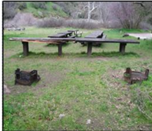
Group site picnic tables are broken and missing parts. Remaining pieces are jagged, presenting visitor safety issues. Currently, there are no fire rings that meet ADA guidelines.
