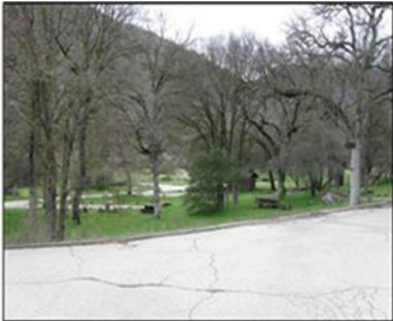
Road is cracking and needs repairs
