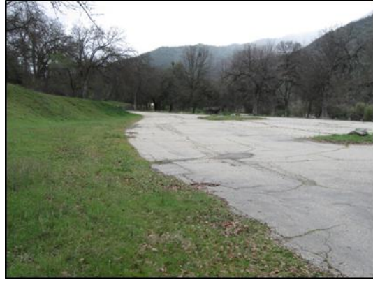
Overflow parking lot pavement is cracked and has several potholes.
