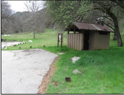
Wood barriers are missing, rotting, and need to be replaced. Bathroom roof is deteriorating.
