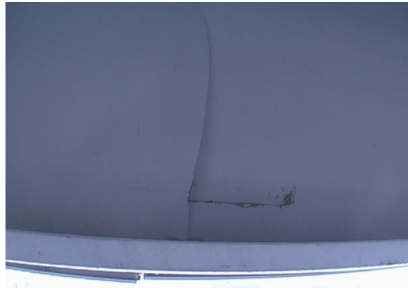
Figure 4-5: Fracture in girder D (Wright, 2000).
