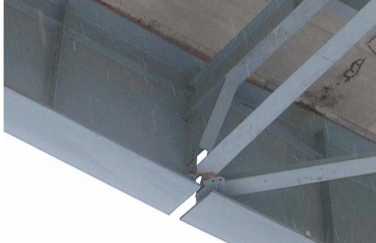
Figure 4-7: Fracture in girder F (Wright, 2000).
