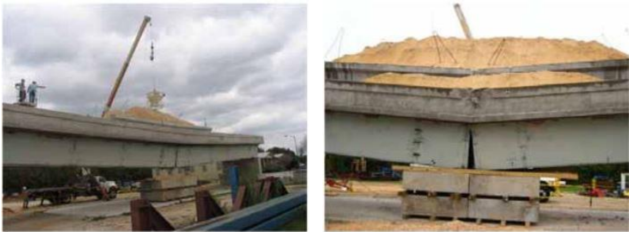
(a) Loading process
