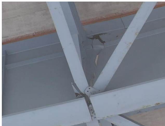
Figure 4-6: Fracture in girder E (Wright, 2000).
