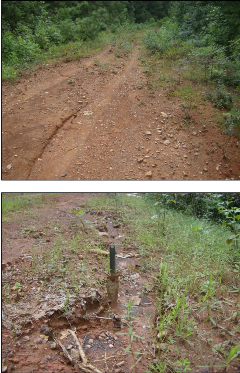
Figure 2.5. Photographs of the most erosive approach displaying an 8 cm deep erosion rill.
