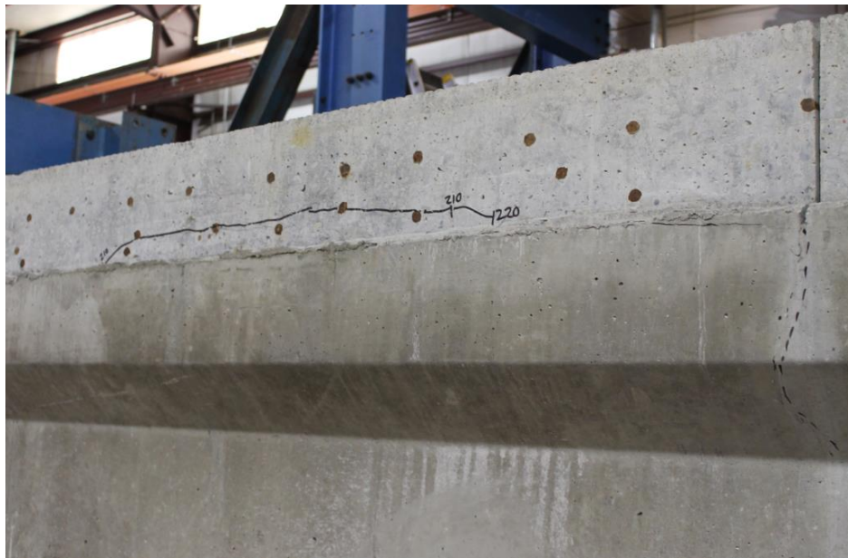
Figure 112- Test 5 Horizontal Shear Transfer Failure
