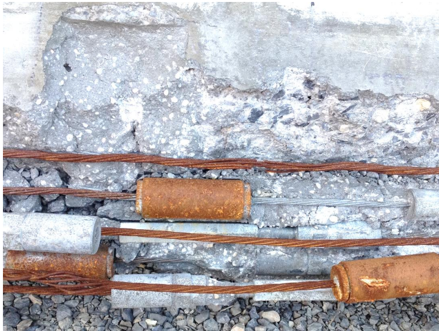
Figure 105- Test 2 Failed Splice and Ruptured Strand
