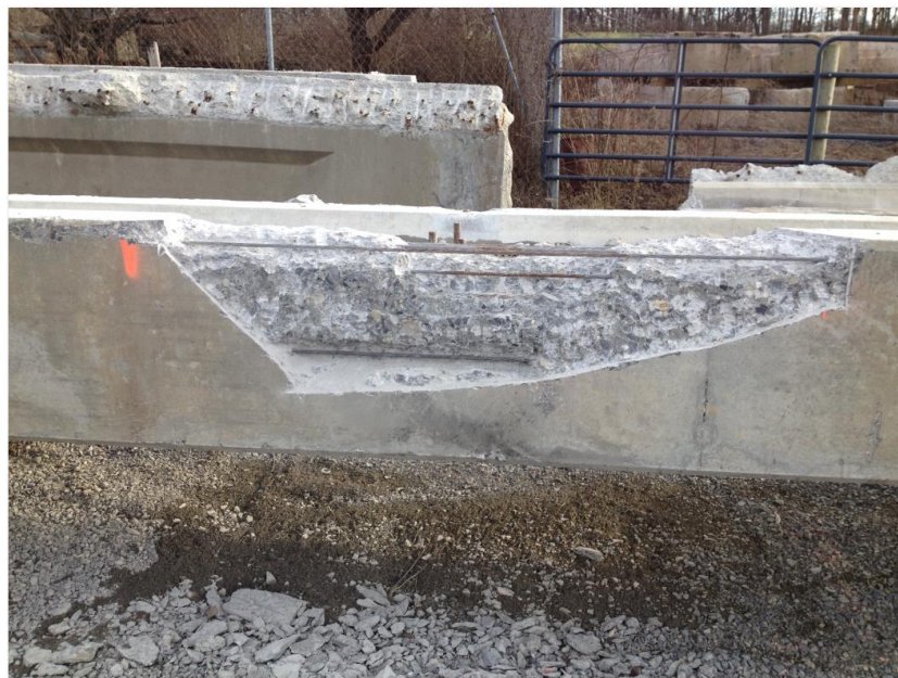
Figure 82- Test 6 Repair area after Damage
