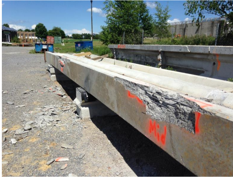
Figure 48- Girder C after Damage from Hydraulic Hammer
