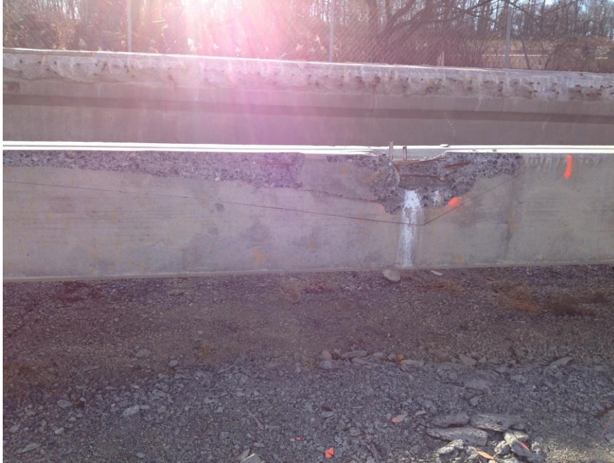
Figure 65- Girder D after Damage from Hydraulic Hammer
