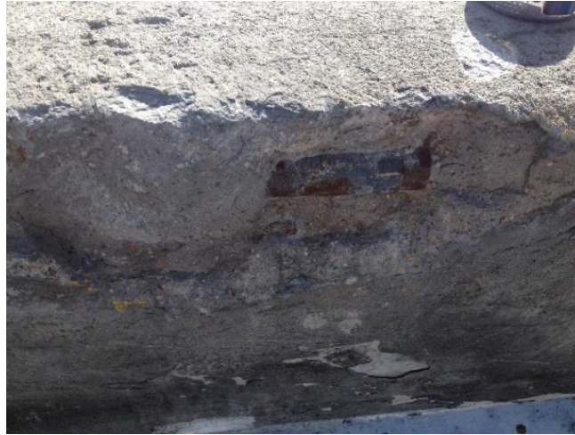
Figure 27- Spall with Exposed Strand Splice Chuck
