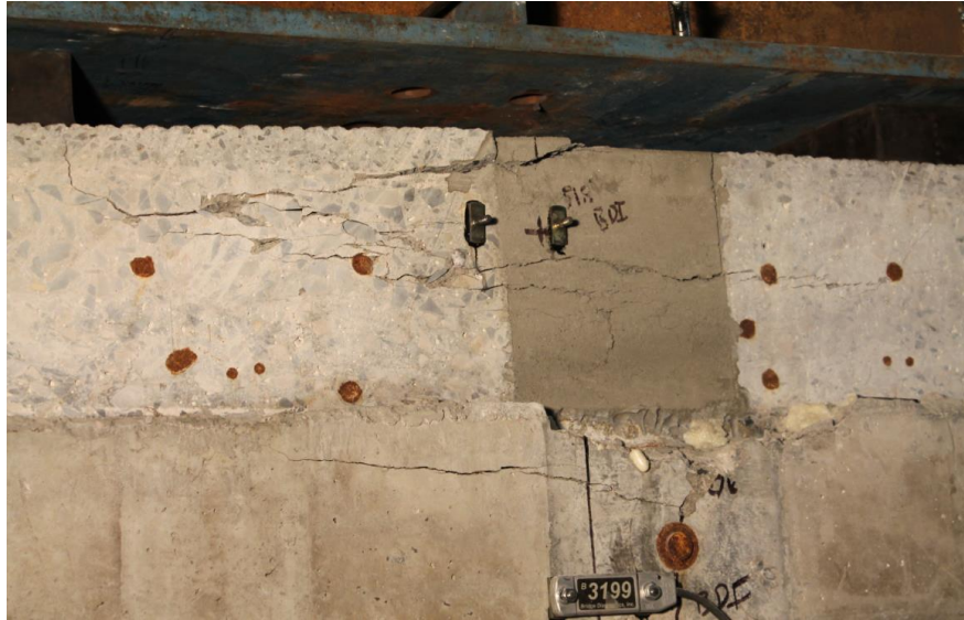
Figure 116- Compression Failure in the Composite Deck
