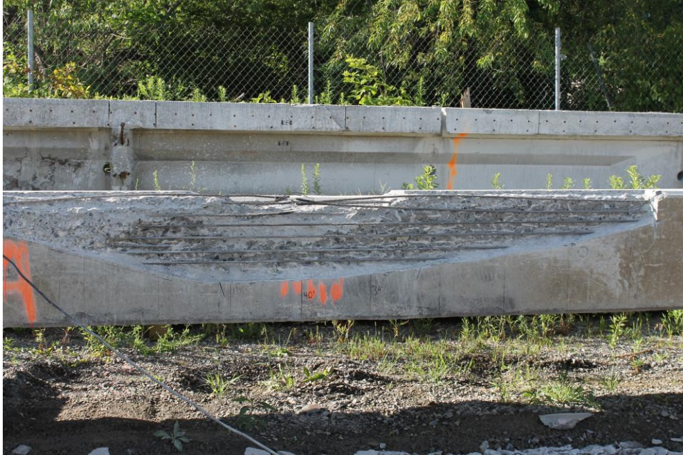
Figure 49- Damage Location for Test 4 Before Repair
