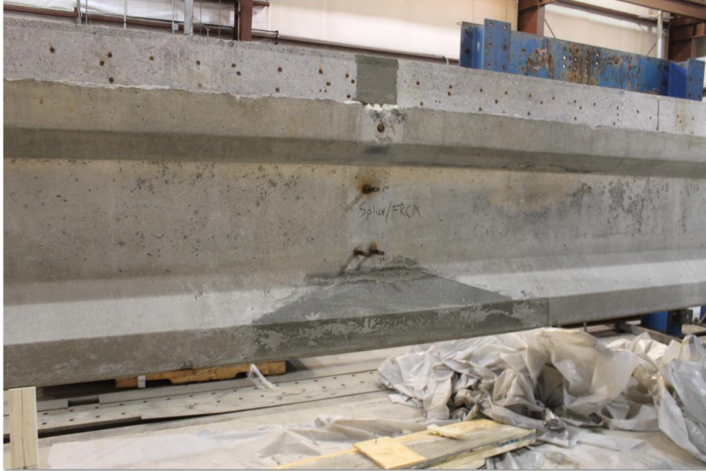
Figure 85- Damage Location after Removal of Formwork
