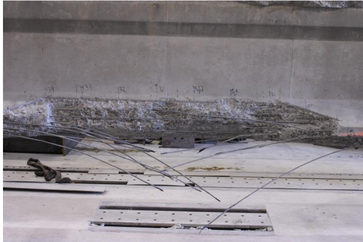
Figure 36- Damage of Girder B Before Repair
