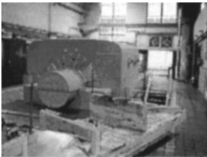
FIGURE 16 Location of outboard generator.
