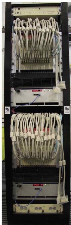
Figure 53. Rack containing two of the nine MicroBooNE TPC readout crates.
