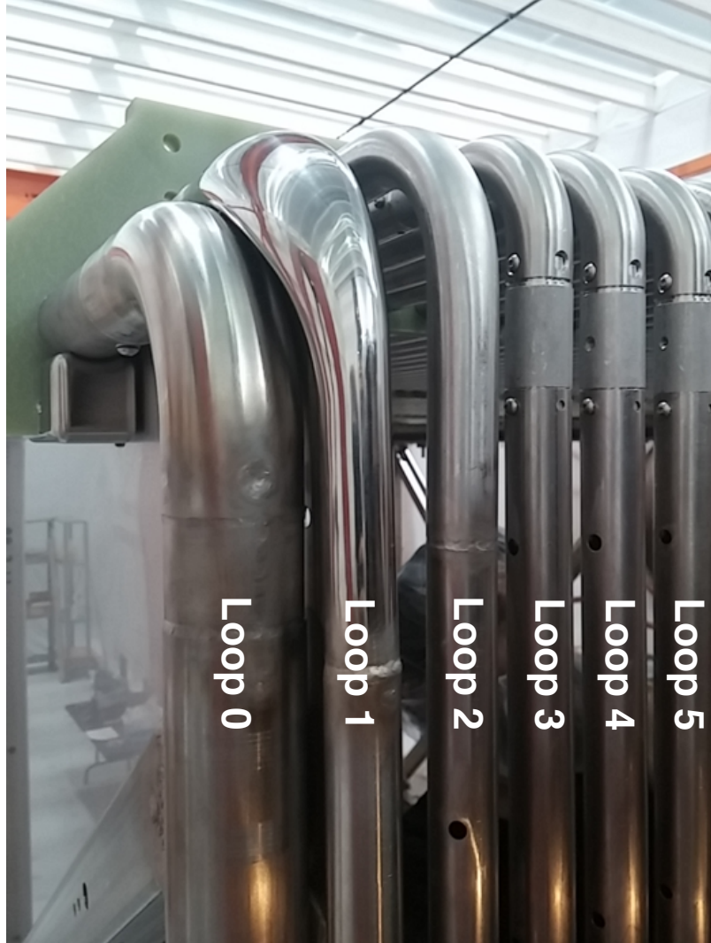
Figure 12. Photograph of the field cage during construction, with loops 0 (cathode) through 5 labeled. Field cage loops closest to (and including) the cathode are modified to reduce sharp edges that would result in higher electric fields.
