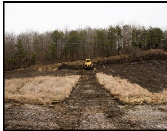
Figure 4. A bulldozer is scraping IES off a site in preparation for tree-planting. This approach may reduce future IES pressure by removing much of the soil seedbank.
