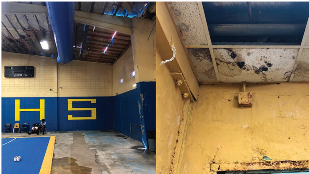
Figure 11.2 Examples of Damaged School Facilities Still in Use
