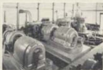
TURBO GENERATOR/ APPALACHIAN POWER CO.
