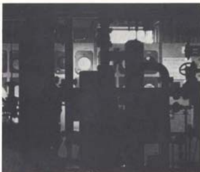
The intricate pipe network in the Chemical Engineering labs.
