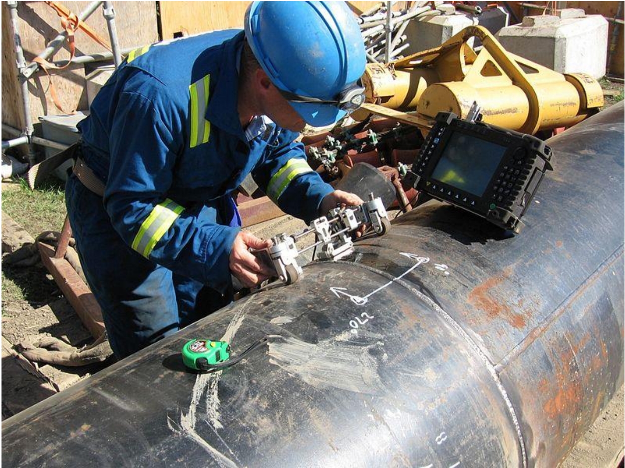
Figure 11 - A technician checks a pipeline using an ultrasonic phased array for weld defects [Public Domain].
