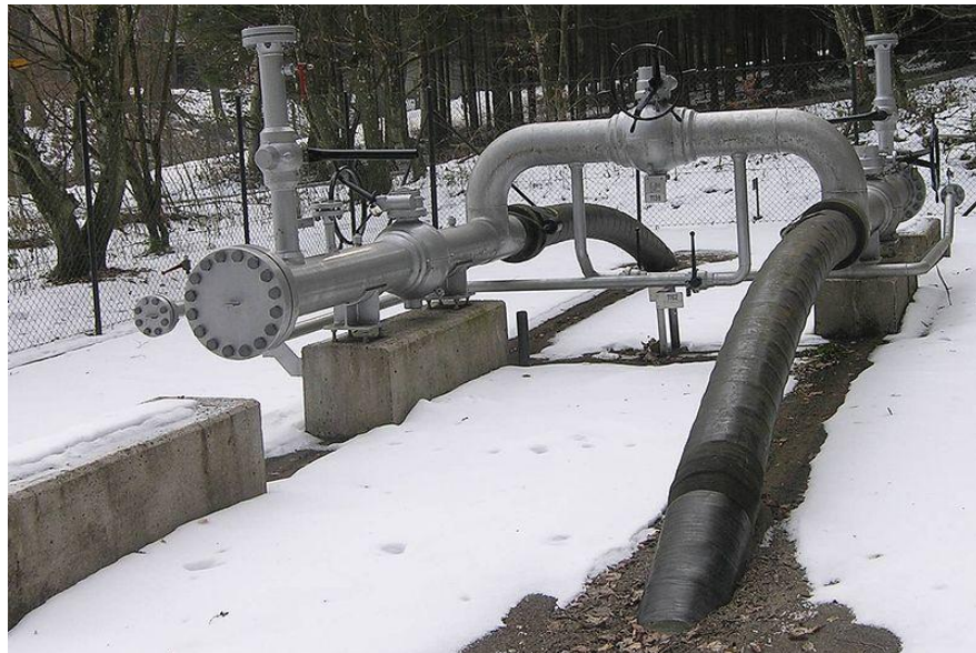
Figure 7 - Pig launcher/receiver utilized by a natural gas pipeline in Switzerland [GNU Free Documentation License – photographed by Audrius Meskauskas]
