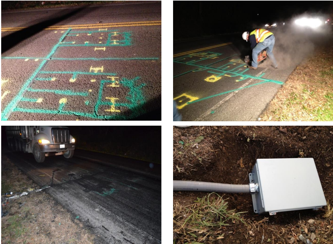
Figure 12: Installation process (a. marking, b. cutting, c. paver passing, d. output cable management)
