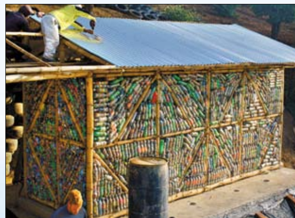
A worker secures the roof above four composting latrines built from plastic trash bottles, bamboo, and chicken wire on top of a concrete slab. The nutrients in the organic waste are absorbed and assimilated on the property.
