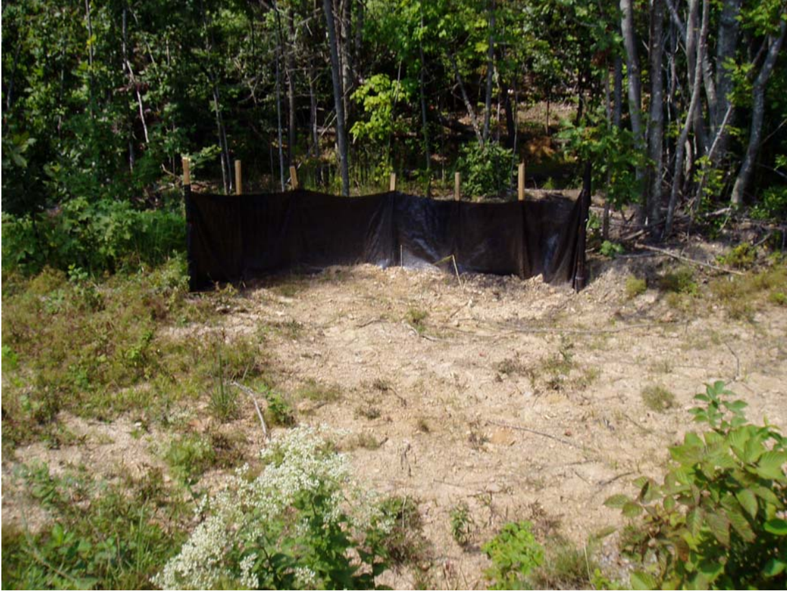
Figure 4-8. A sediment trap receiving surface flows from a cutover area and revegetated fireline but not receiving flows directly from any roads in Central Virginia.
