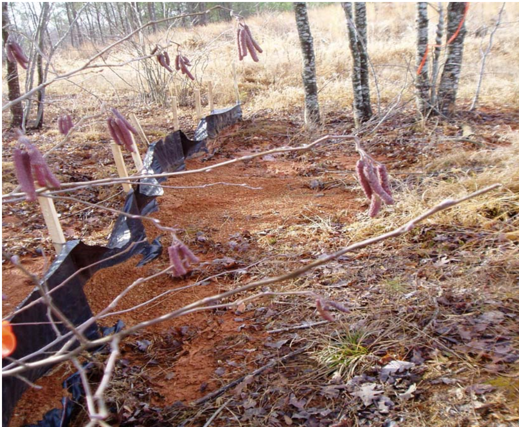
Figure 4-7. A sediment trap receiving large sediment loads directly from a failed water turnout on a forest road in central Virginia. Distance to the road is approximately 3 chains or 200 feet.
