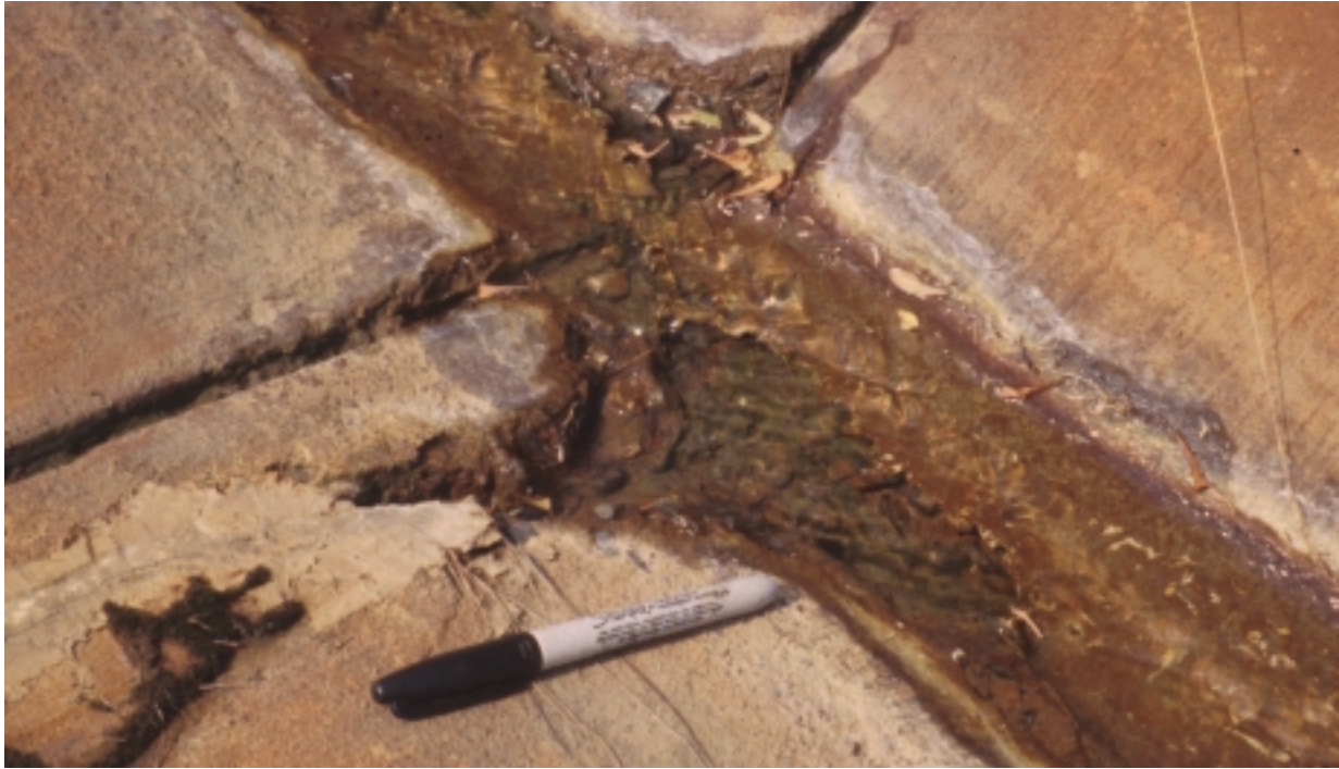
Figure 3.6. Acid drainage from the Quantico slate Stafford, Virginia, (see Figure 1.1) has caused extensive iron staining and concrete etching along the curbs and sidewalks of the Hampton Oaks subdivision.
