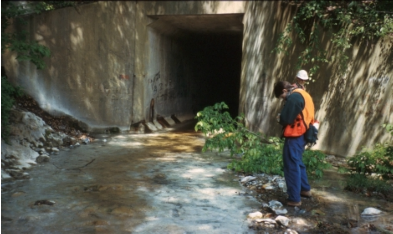
Figure 3.9. Acid drainage from the Millboro shale, exposed along I-64 in Clifton Forge, has decimated this stream. The pH of water samples from the downstream end of the culvert has ranged from 2.9 to 7.1. Iron and aluminum precipitates coat the stream bed, and concrete joints within the culvert have been degraded.
