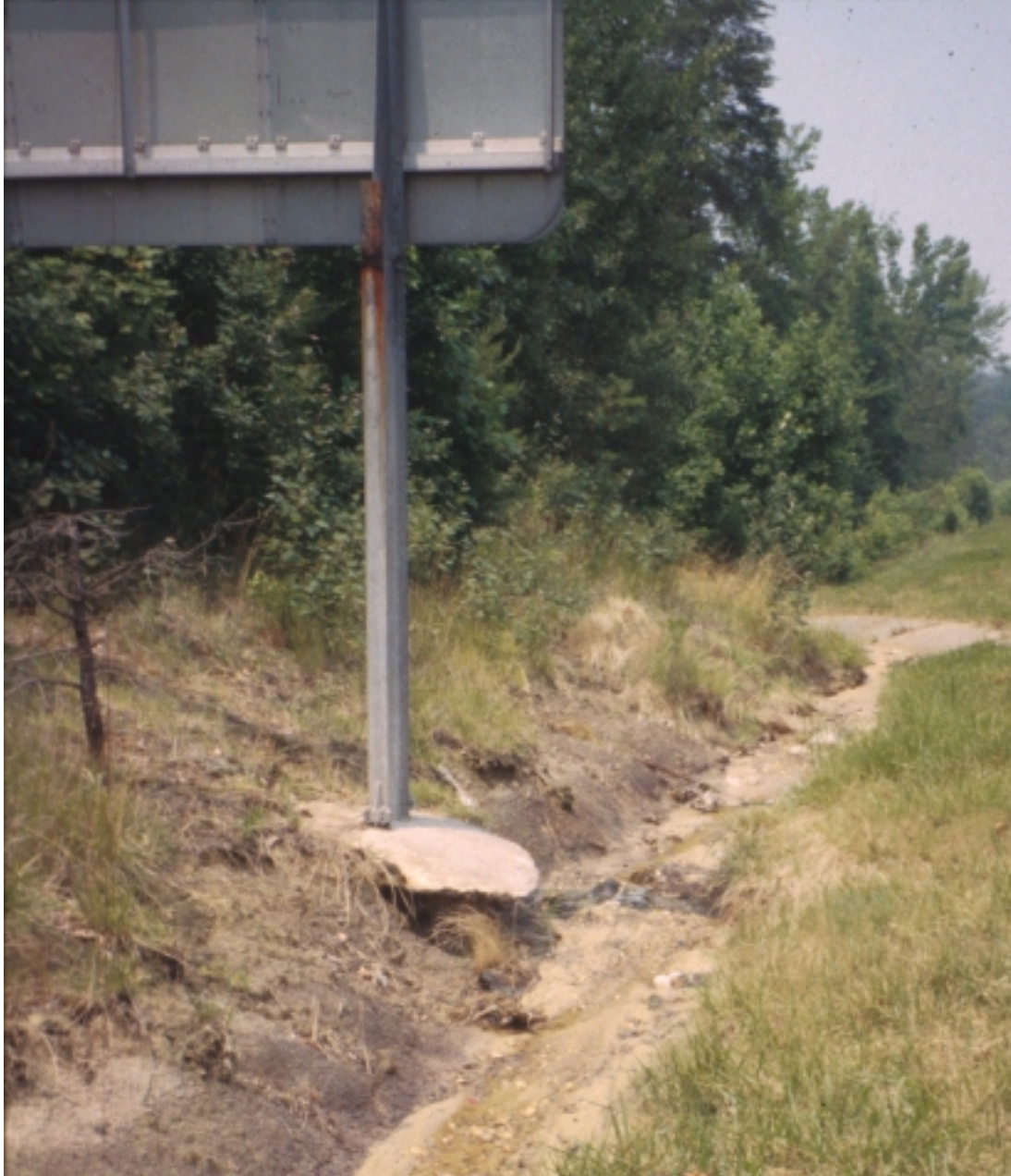
Figure 1.1. Sulfide-bearing sediments of the Chesapeake Group are exposed along this stretch of I-95 in Spotsylvania County. The stability of this signpost is compromised due to concrete degradation from acid attack. Furthermore, acid conditions (soil pH \sim 2.5) limit vegetative growth, which makes these sites particularly prone to erosion.
