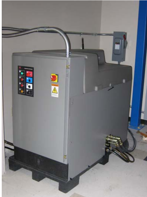
Figure 3-13 MTS SilentFlo Hydraulic Power Supply
