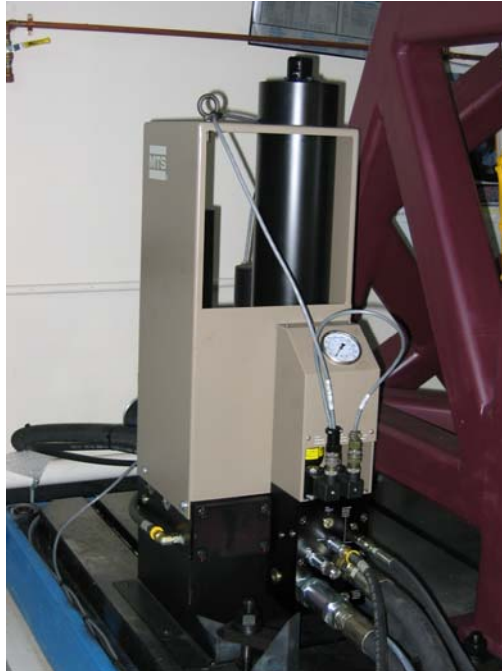
Figure 3-14 MTS Hydraulic Service Manifold
