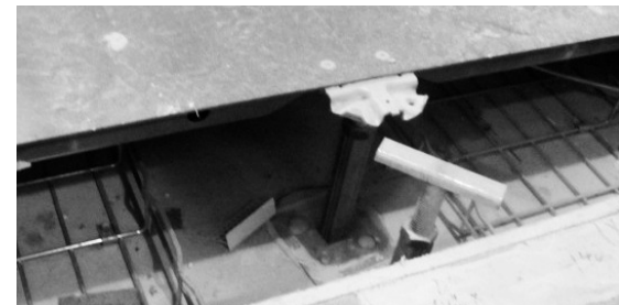
Figure 3.4.2.1 (top): Steel structure is fabricated in-house by company employees before being moved outside and installed on a temporary foundation.
