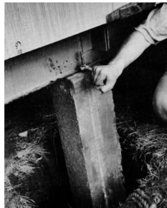
Figure 2.6.4.2 Acorn House foundation installation: The steel chassis sub-floor structure rests on a cast-in-place concrete pier foundation located directly beneath the central core (Koch 1958, 93).
