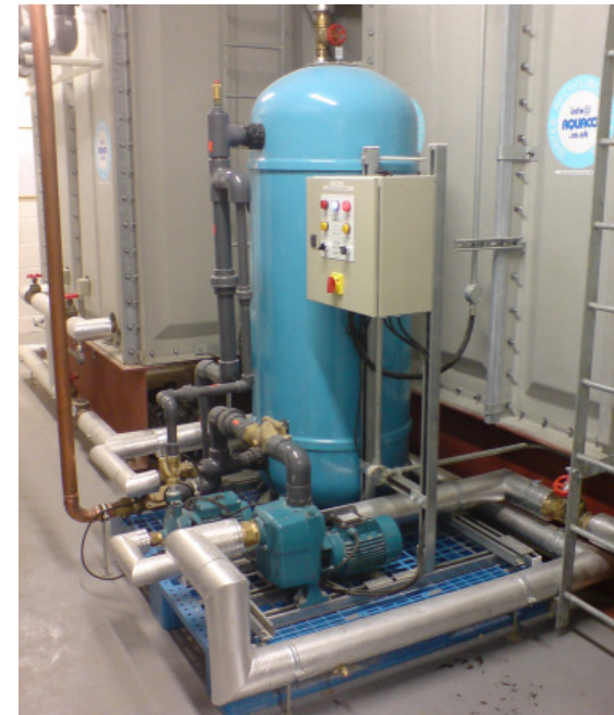
Figure A.10 grey water purification system (Aquaco Grey Water Recycling System 2010)
