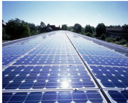
Figure A.12 photovoltaic array (Applied Solar Technology 2012)
