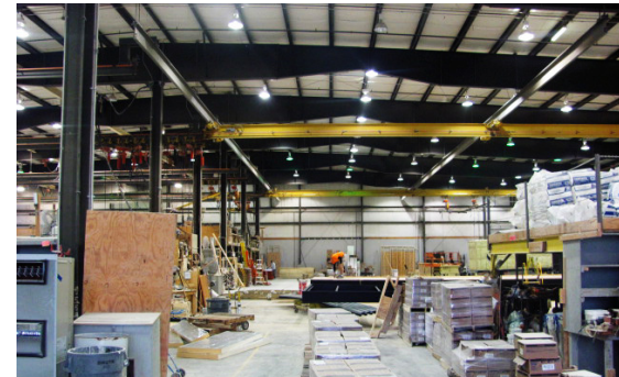
Figure 3.4.1.2: Overhead pulleys/jigs installed throughout the factory for the handling of floor panels, wall segments, and roof components.
