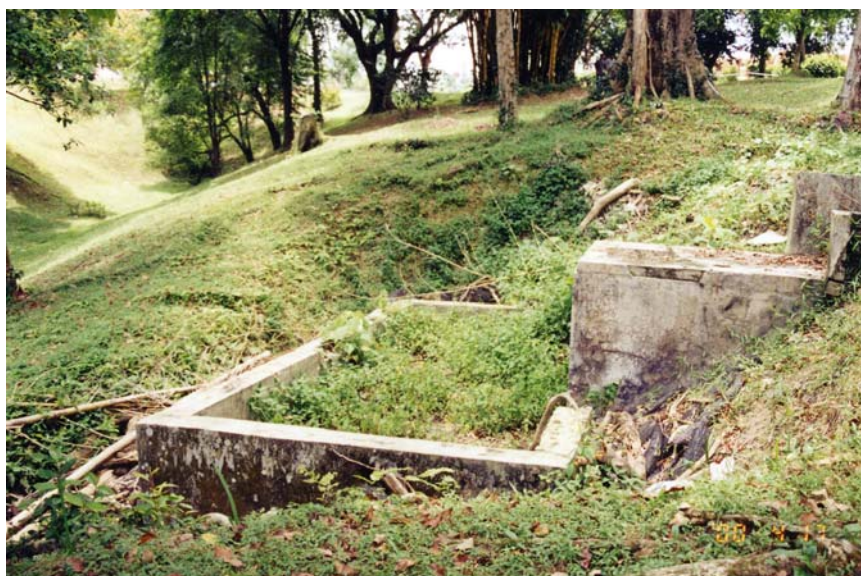
Figure 7. Park drain system that has deteriorated
