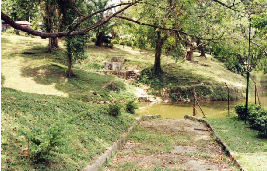
Figure 8. Park drain system that has deteriorated
