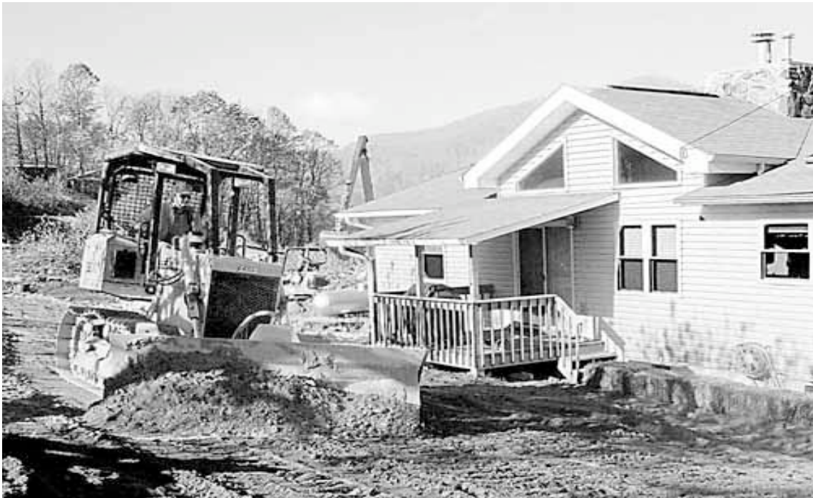
Fig. 12. A bulldozer removes soil from a yard at Barber Orchard in Haywood County, North Carolina in 1999 – © 2000 Raleigh News & Observer. This process was part of the cleanup provided by the EPA during the emergency removal action in 1999-2000.
