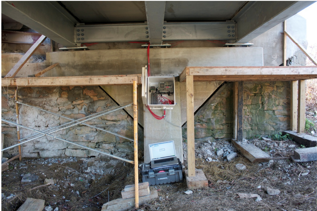
Figure 3-13. Photograph of CR23X data logger on the western back wall
