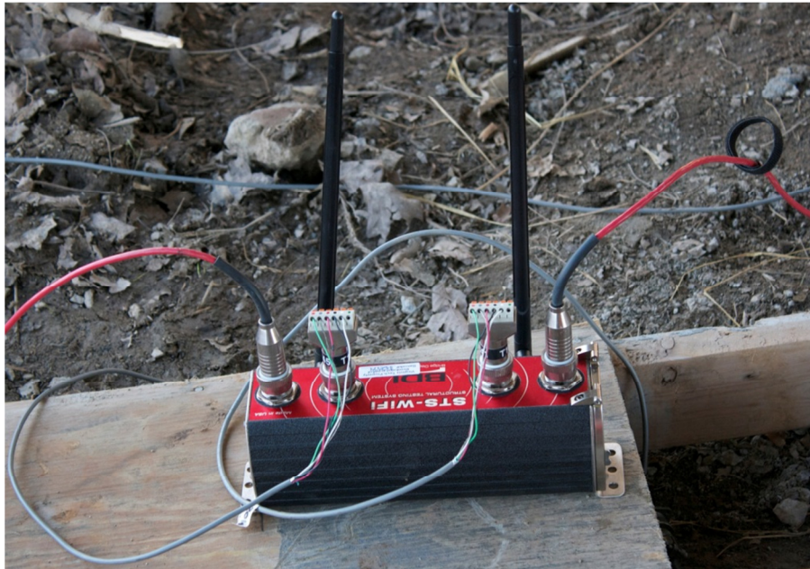
Figure 3-21. Photograph of a STS-Wifi Node
