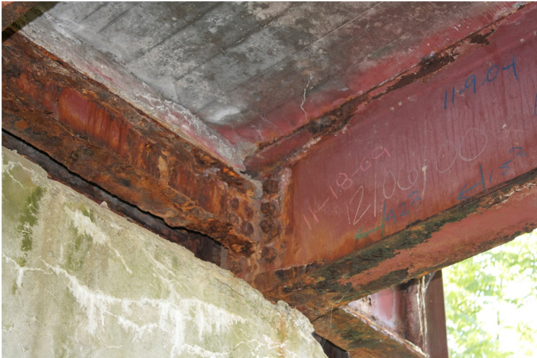
Figure 1-2. Photograph of the Corrosion at the Joints between Spans
