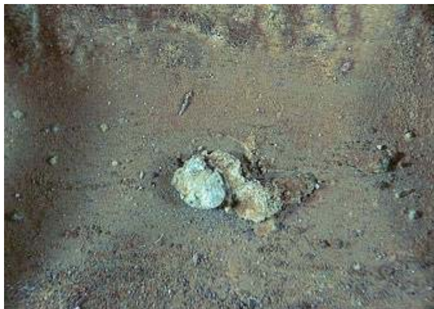
Figure 1-3 A large isolated pit on WSSC residential copper tubing typical of the type used to develop polarization scans. The mound, or tubercle, is formed by rapid copper corrosion underneath the pit.
