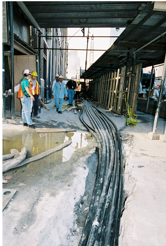
Figure 3 – Above ground cables provided temporary service following 9/11.
