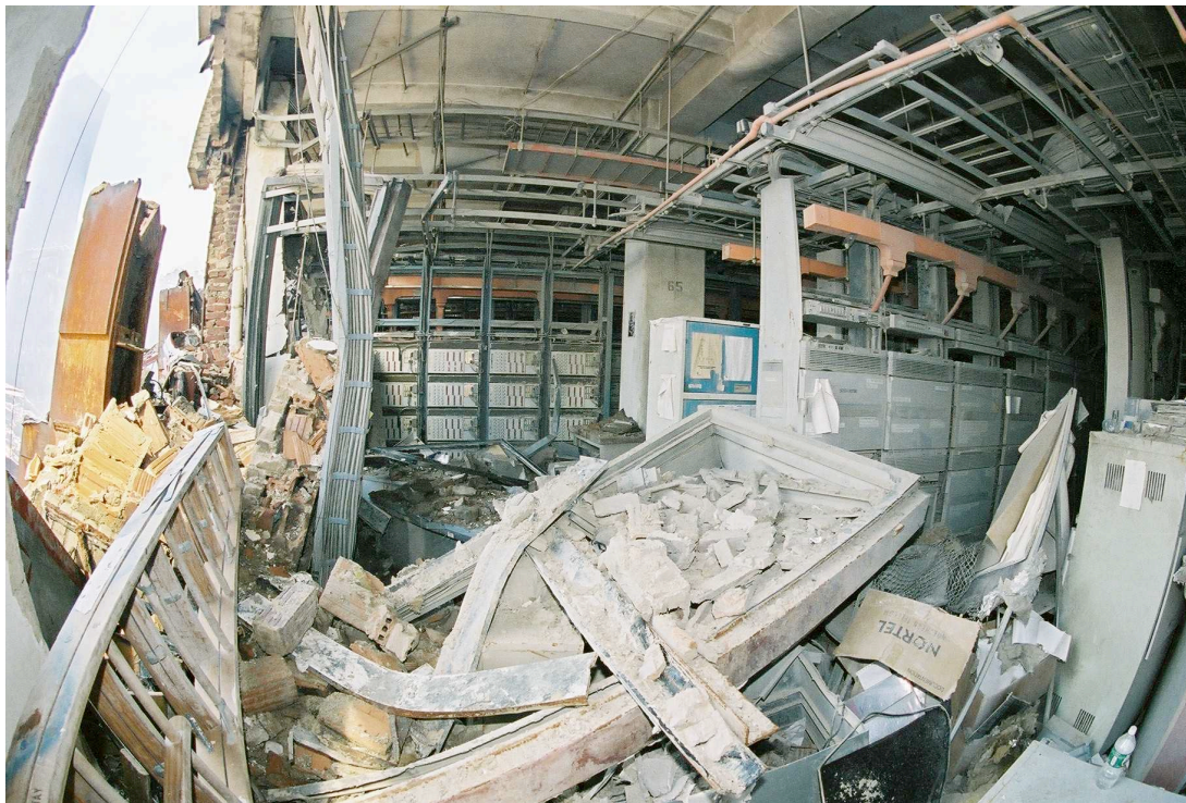
Figure 2 – Damage inside the facility.
