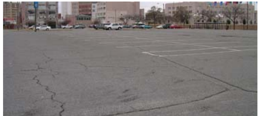
Figure 5.3. Example Parking Lot in Norfolk, VA. This existing municipal parking lot illustrates the need for the regulation and enforcement of ordinance requirements.
