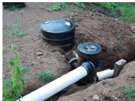
Figure 9. Underground storage tank
