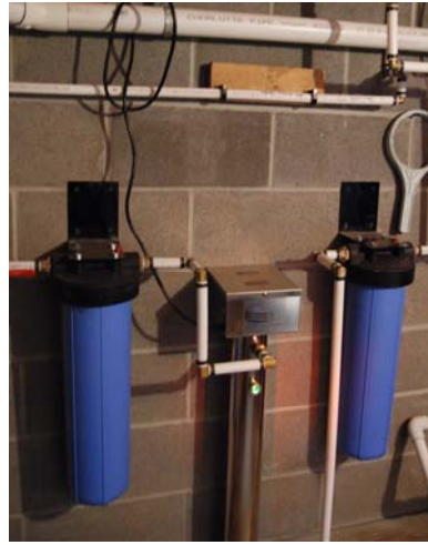
Figure 6. UV light treatment unit
