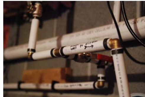
Figure 8. Pipe and valves for dual operation
