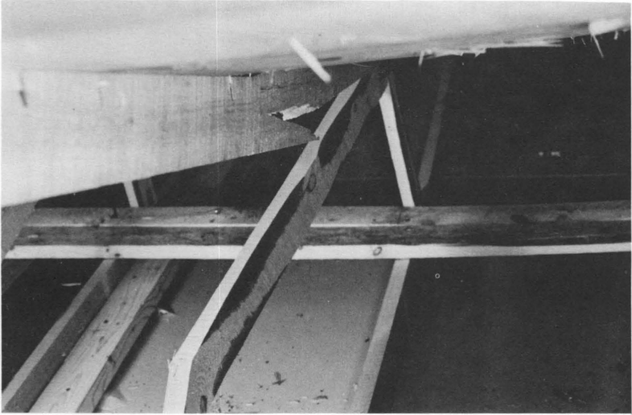
Fig. 18. A TYPICAL ROOF TRUSS FAILURE
