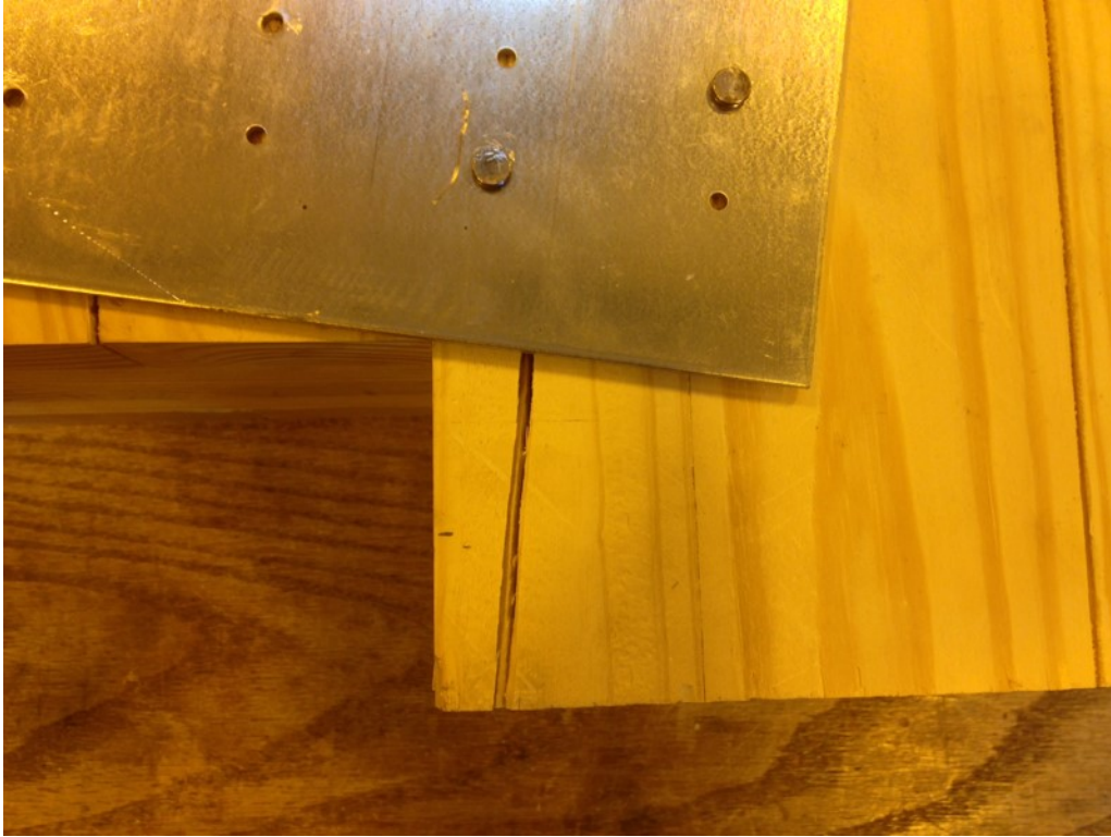
Figure 4-16: Photograph of Wood Splitting Failure in M-SS-5
