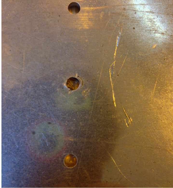
Figure 4-18: Elongation of Nail Holes in the Steel Plate
