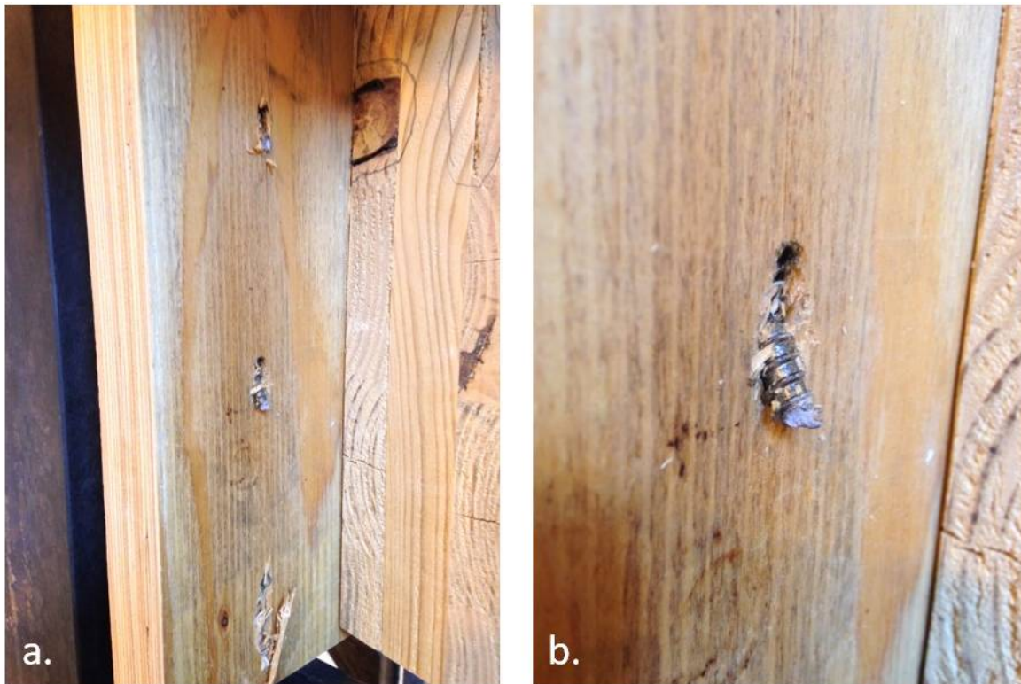
Figure 4-7: Photographs of Observed Failure in M-SS-2
