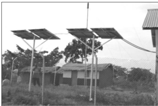
Solar photovoltaic panels outside a secondary school at the Bukasa demonstration site (Lake Victoria, Uganda).
