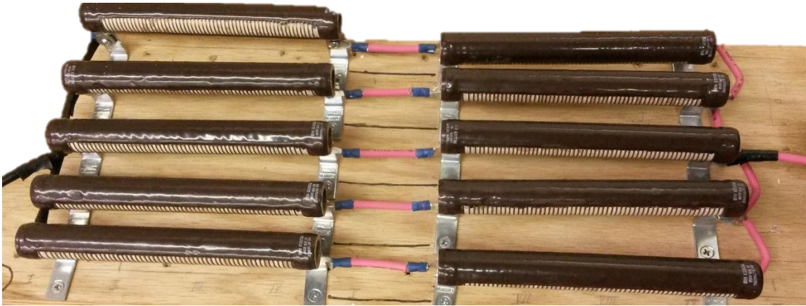
Figure 5.10 Low amperage resistor setup. Five parallel branches of two, 1 \Omega 100 \text{ W} resistors.
