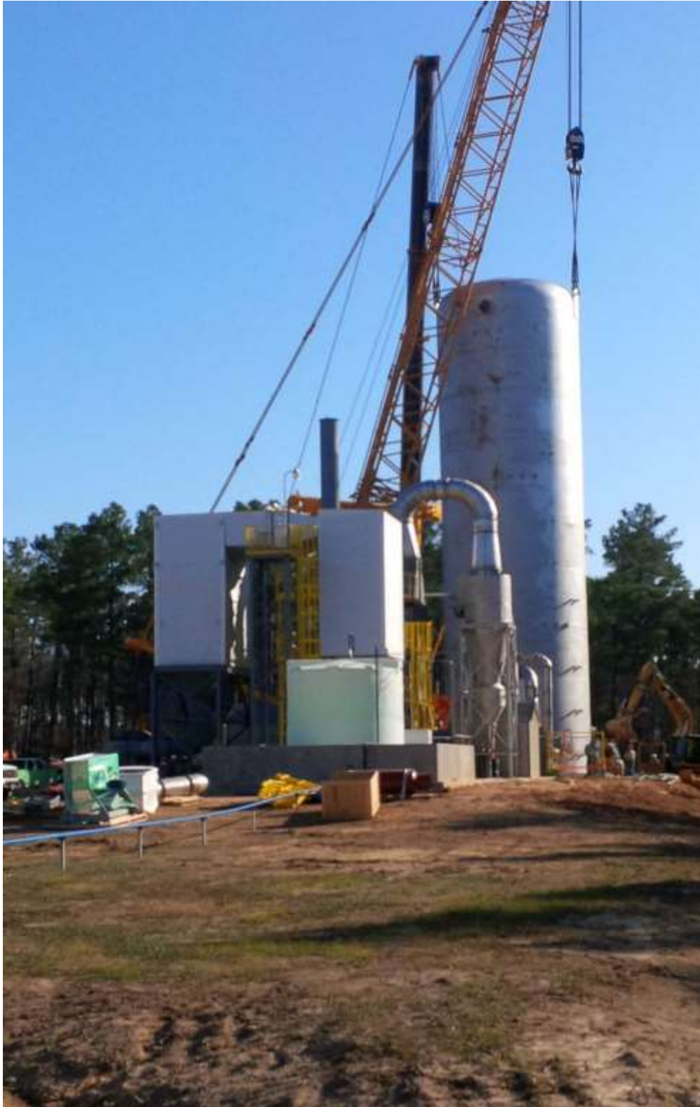
Figure 56: The Contained Burn Structure with the Pollution Abatement System 547
