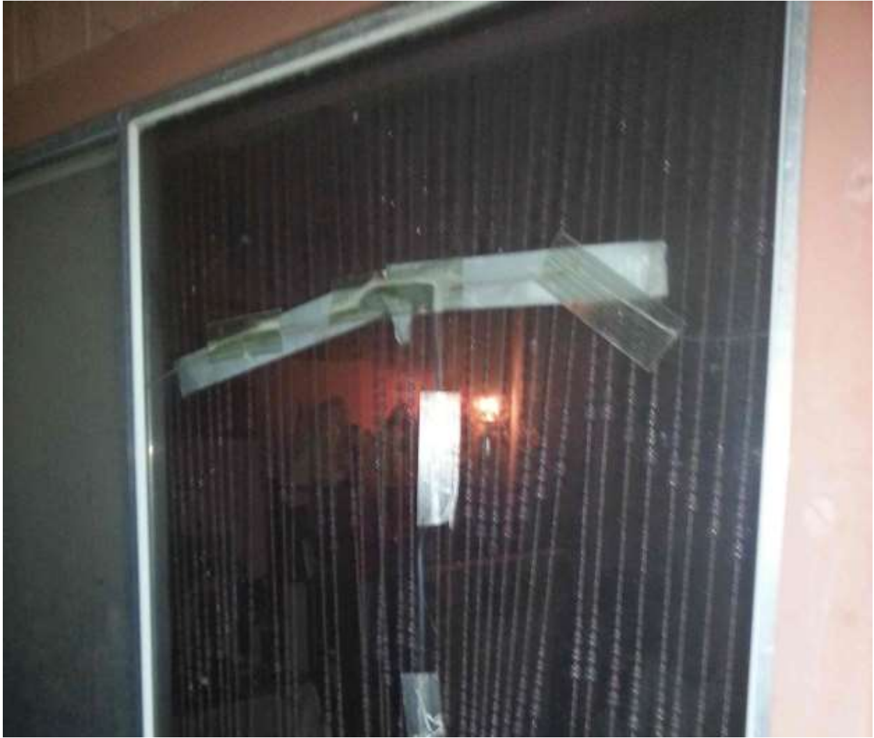
Figure 5: Damage to Fenceline Home from Blasting on the fenceline; No Electricity in Home Next to Mine Providing Electricity
