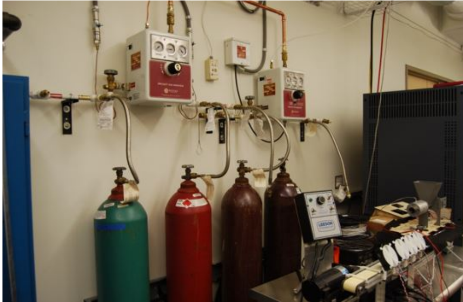
Figure 3.8: The hydrogen and argon gas bottles and regulators used to supply the kiln to sinter the binder jetted pieces.
