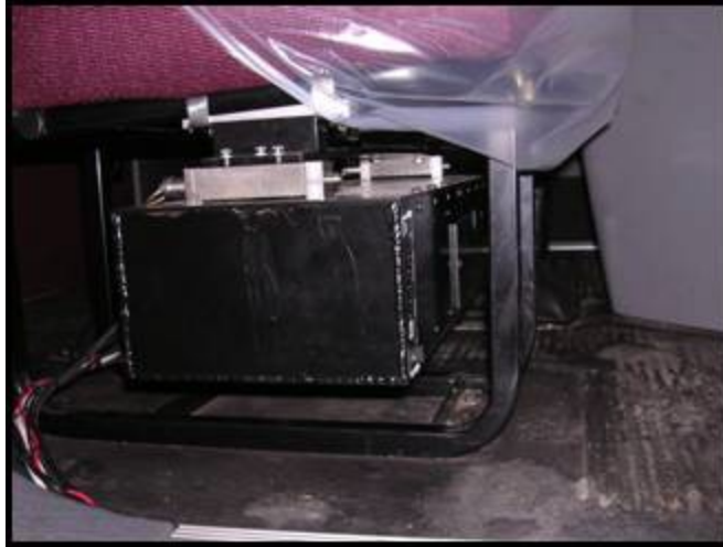
Figure 1. Photo. Encased computer and external hard drive installed under the passenger seat.
