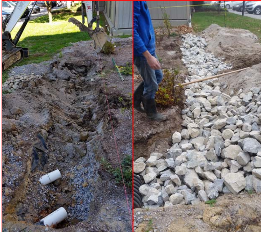
Figure 12. Excavation of bioretention cell and installation of riprap improve flow into BMP.
