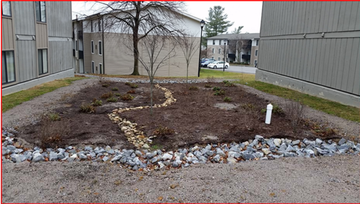
Figure 14. Final retrofitted bioretention cell. We will incorporate topsoil and grass during the spring of 1017.
