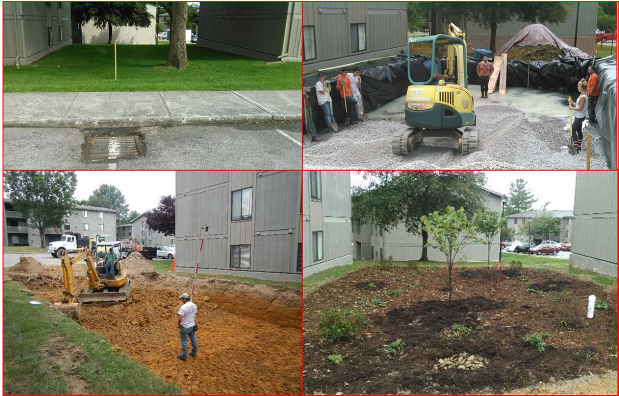
Figure 11. Installation of large bioretention cell at Foxridge Apartments in 2015. Images show before, during and after construction.
