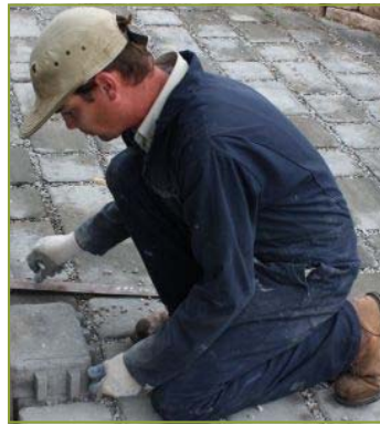
"Measure twice, cut once." Paul Chumbley sizes up a Techo Bloc® paver. Photo H. L. Scoggins.
