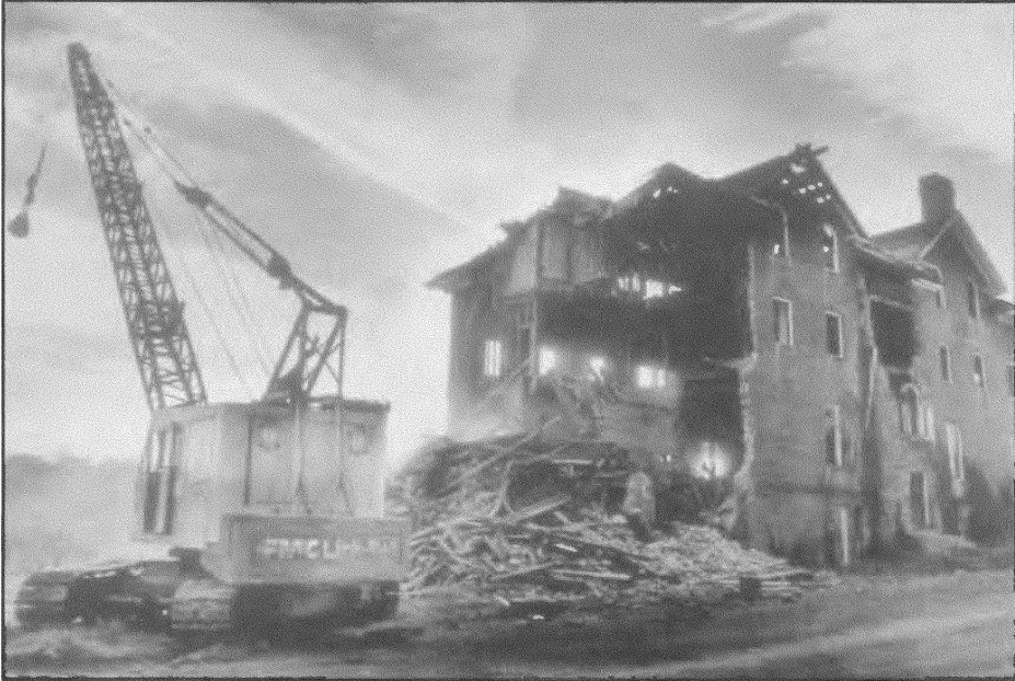
Baily Morris Hall, completed in 1912, met its destruction in 1980 by wrecking ball, the outcome of a local public policy decision. (Photograph by Gene Dalton, Roanoke Times staff photographer; photograph courtesy of The Roanoke Times)
