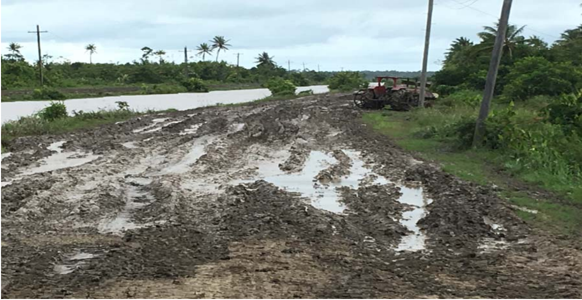
Figure 6.1 Poor condition of access dam
