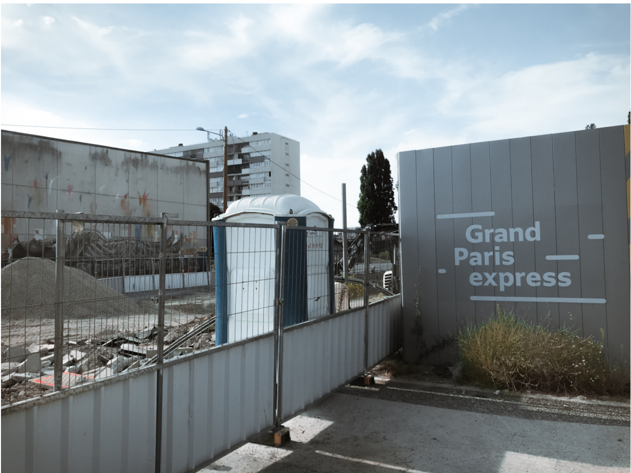
Figure 2: Construction site for line 16 of the Grand Paris Express, Montfermeil in Seine-Saint-Denis (The future station will be located at the border of two suburban towns: Montfermeil and Clichy. The construction started in 2016 and is scheduled to be completed by 2024). (Source: GEFFROY; Date: June 2018)
