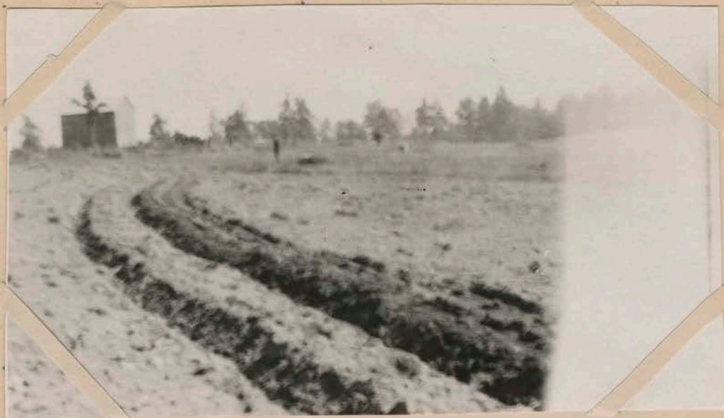
Fig. 4. A broad-base terrace under construction Note grade furrow on upper side plowed out first.
