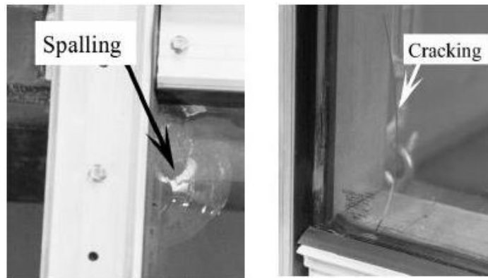
a) Glass spalling and cracking occurring at the corner regions (vision areas) (Memari et al. 2011a)
