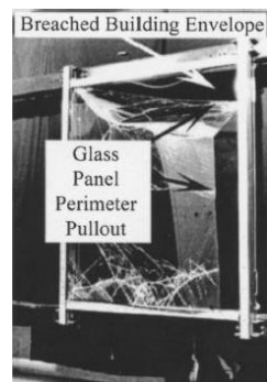
a) Glass pullout damage state observed in a laminate glass unit CW system (Memari et al. 2003)
