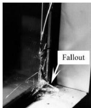
Figure 2-20: Glass fallout damage state in vision area of glass CW specimen (Memari et al. 2011a)
