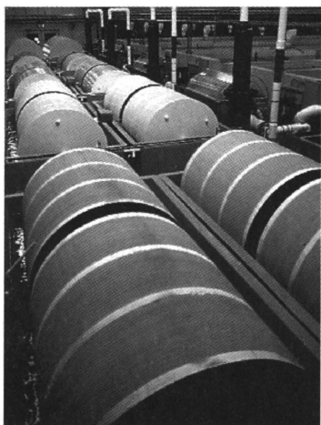
System #1 – RBCs servicing 115,000-liter cross-flow raceways.
