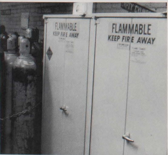
146. Hazardous material storage
