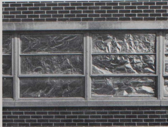
73. Dysfunction - inadequate sun control
