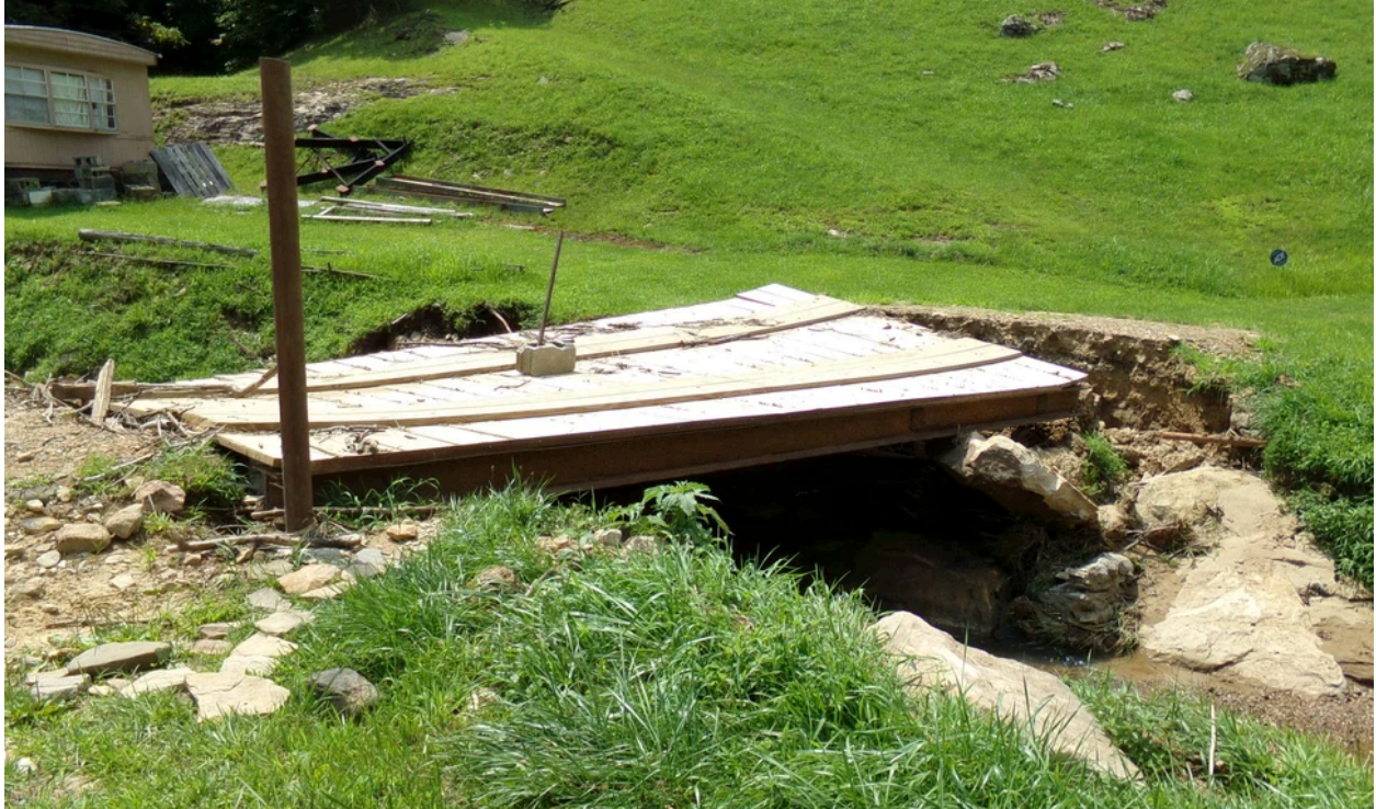
Figure 1: Private Access Bridge Before WVBHP Replacement (Courtesy of WV VOAD)
