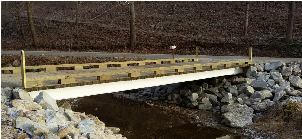
Figure 2: Private Residential Bridge After Bridge Home Program Replacement (Courtesy of WV VOAD)
