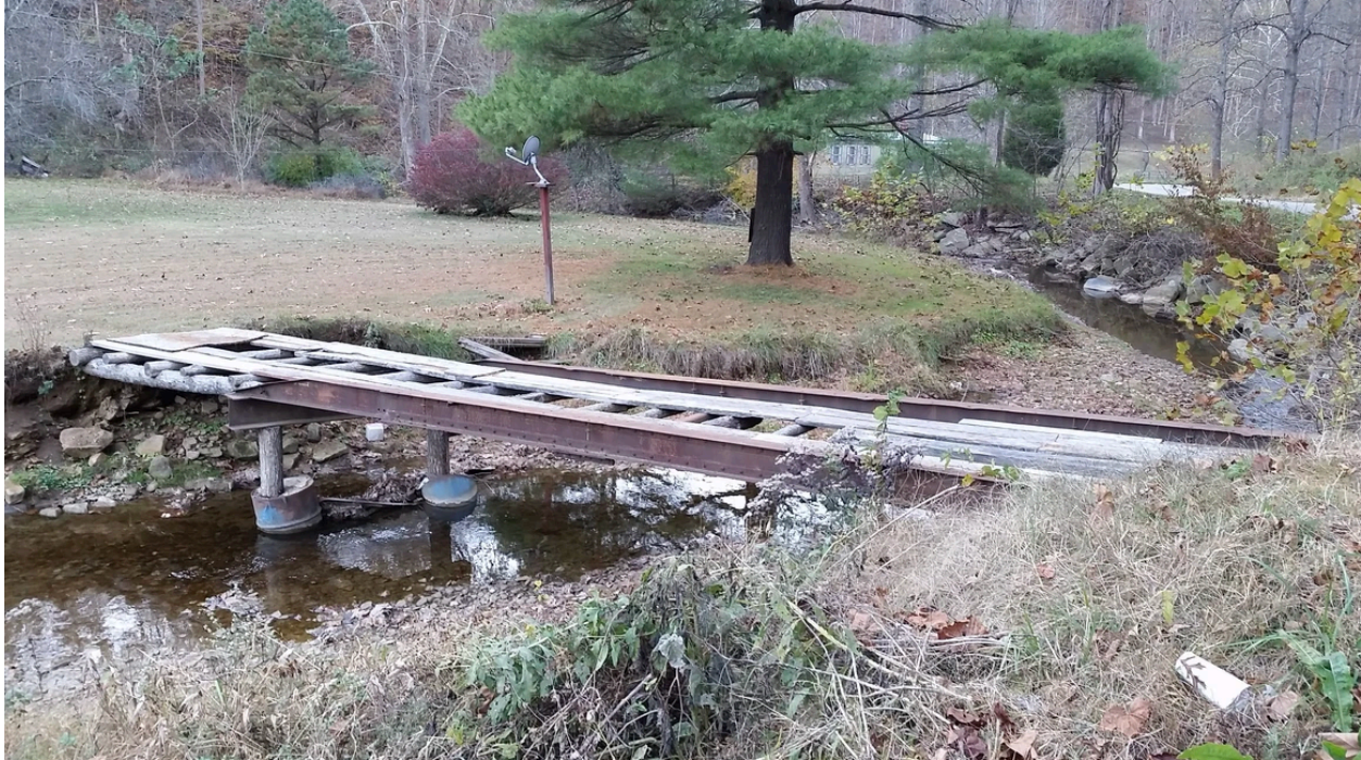
Figure 1: Poorly Designed Private Residential Bridge Before Bridge Home Program Replacement (Courtesy of WV VOAD)
