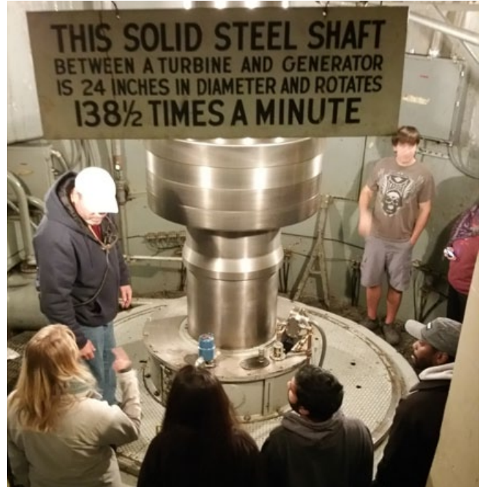
Mr. Richard Palmer of Appalachian Power explains how the hydro-electric turbine generates electricity.
