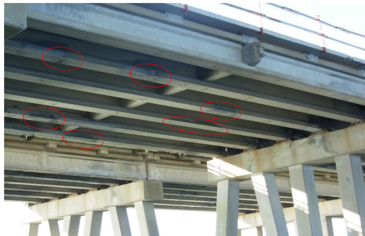
Figure 1.15. Chloride-induced corrosion damage in Lesner Bridge, Virginia [reproduced from (Alfailakawi et al., 2020)].
