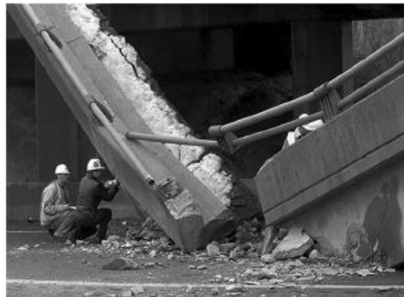
Figure 1.2. Partial collapse of Lake View Drive Bridge due to corrosion [reproduced from (Harries, 2009) ].
