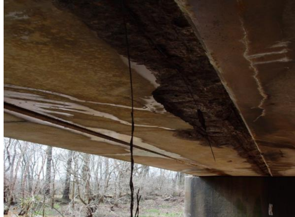
Figure 1.1. Chloride-induced corrosion damage in prestressed bridge girders [reproduced from (Alfailakawi et al., 2020) ].
