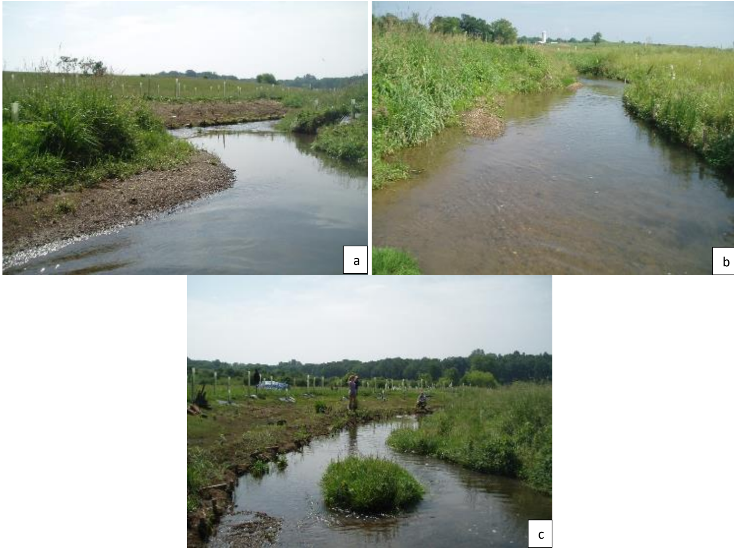
Figure 10: Treatments 2 and 3 during construction. a) Treatment 2 with banks regraded, gravel bars forming; b) Treatment 3 gravel bars forming; c) Treatment 3 with constructed inset floodplain.
