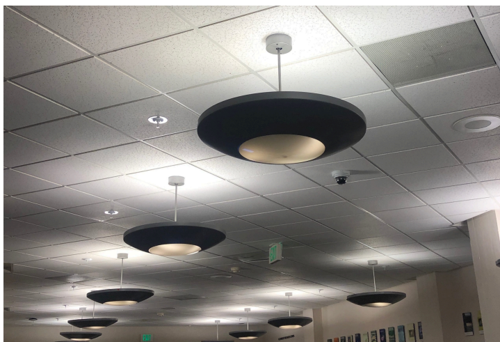
Figure 4.16: Acoustic ceiling tiles example.
