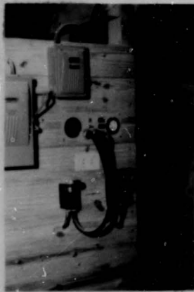
Control panel for the automatic feed grinding, mixing and feeding equipment on the Lilley farm.
