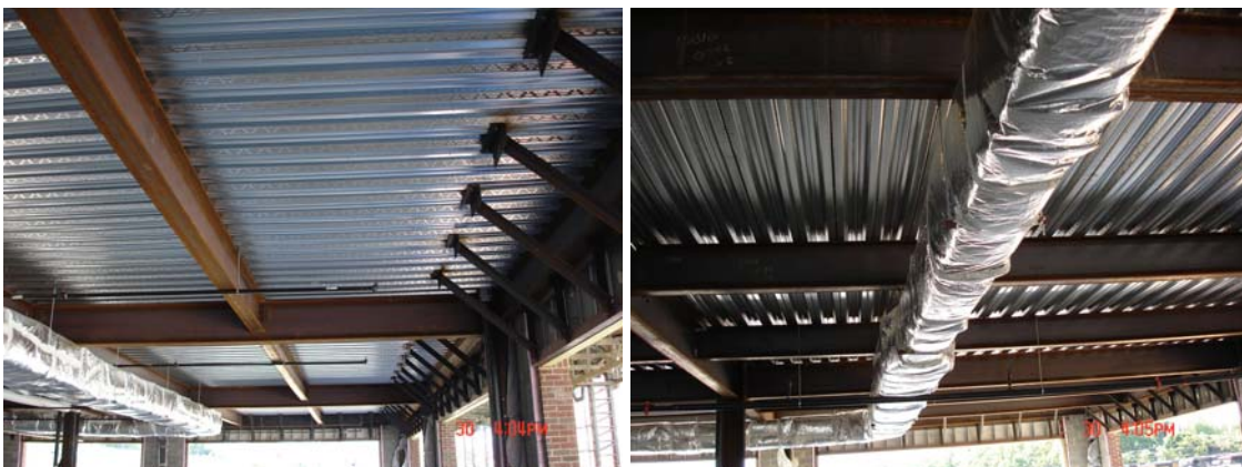
Figure 4.54: Riverside MOB Slab Underside Condition
