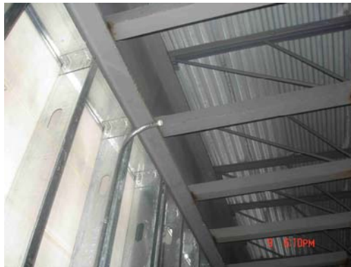
Figure 4.77: First Bank & Trust Building Spandrel Condition
