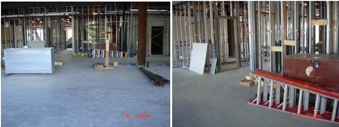
Figure 4.53: Riverside MOB Slab Topside Condition
