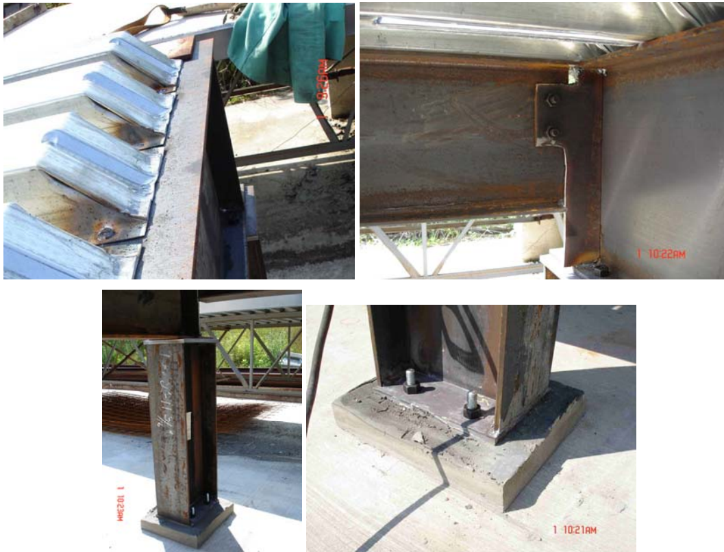
Figure 4.3: Long Span Composite Slab Construction Details. (a) Deck Spot Welds; (b) Beam Connection; (c) Stub Column; (d) Base Plate.
