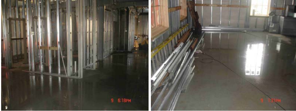
Figure 4.74: First Bank & Trust Building Slab Topside Condition
